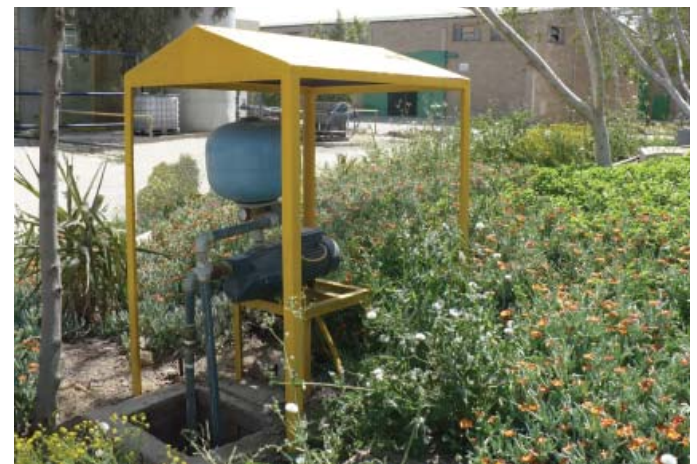
Water pump for irrigation
