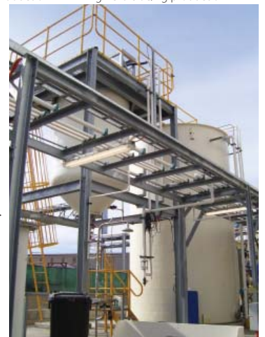
New wastewater storage and treatment plant
