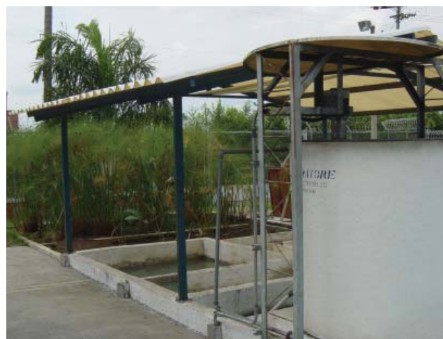
The effluent treatment plant
