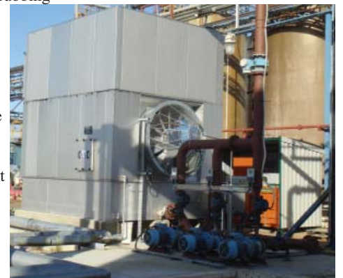
New cooling tower
