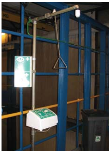
Additional safety shower/eye wash
