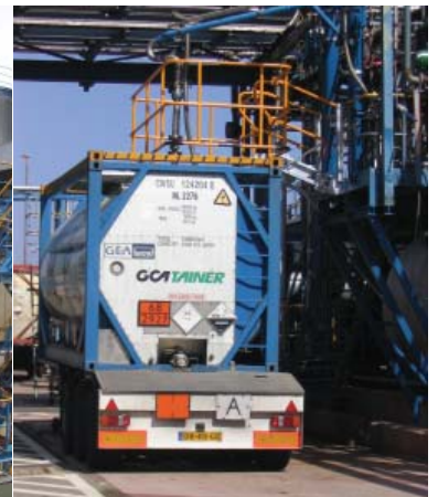
Safety cage for tanker unloading
