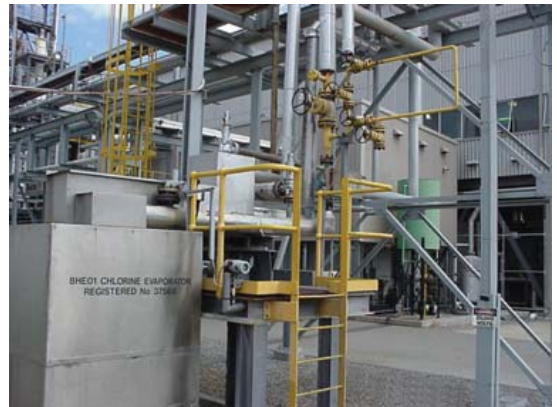
Liquid chlorine storage
